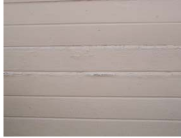
CLASS I PAINT CONDITION
