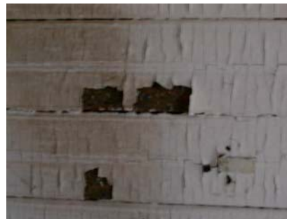
SEVERE CRACKING AND ALLIGATORING PAINT SURFACE, WITH BARE WOOD VISIBLE
