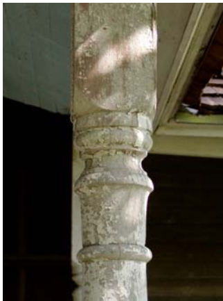
PEELING PAINT DUE TO LACK OF MAINTENANCE
